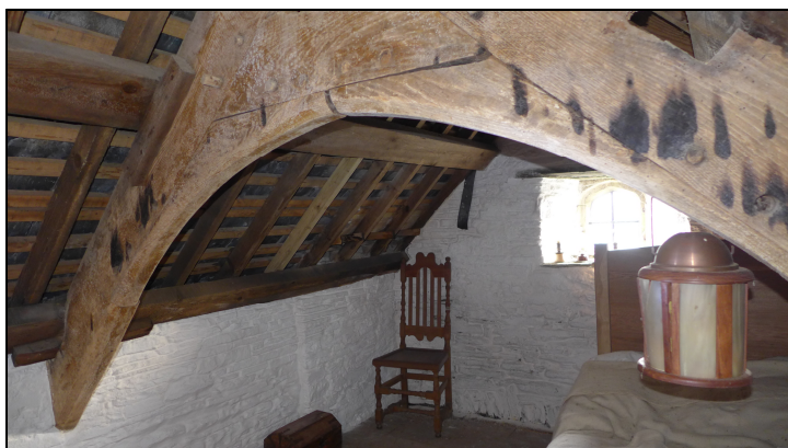
Fig. 7. Llancaiach Fawr Manor burn marks, South Wales
