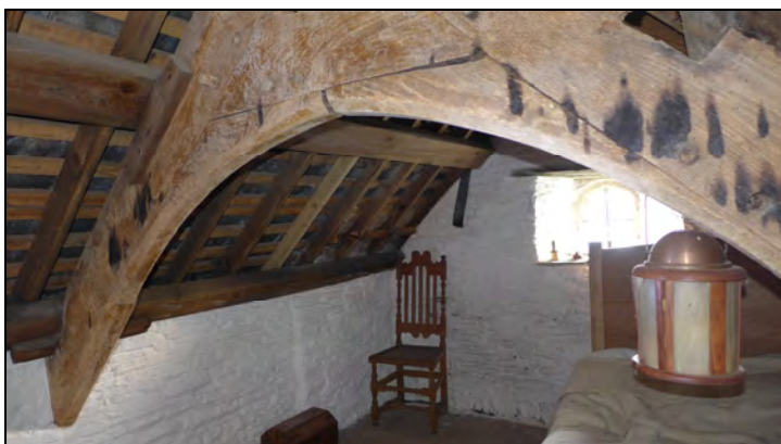
Fig. 7. Llancaiach Fawr Manor burn marks, South Wales
